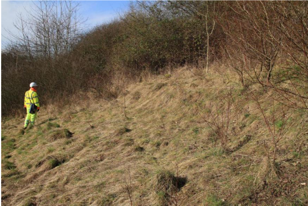
Figure 10: A5 Milton Keynes showing the area immediately below the trial with significant signs of instability (Site Photograph 7DW_4057)
