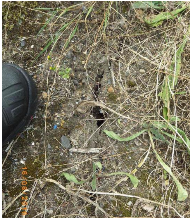
Figure 16: M23 Gatwick trial showing crack at the crest of the embankment (Photograph courtesy and by permission of Martine Mildon, A-one+)
