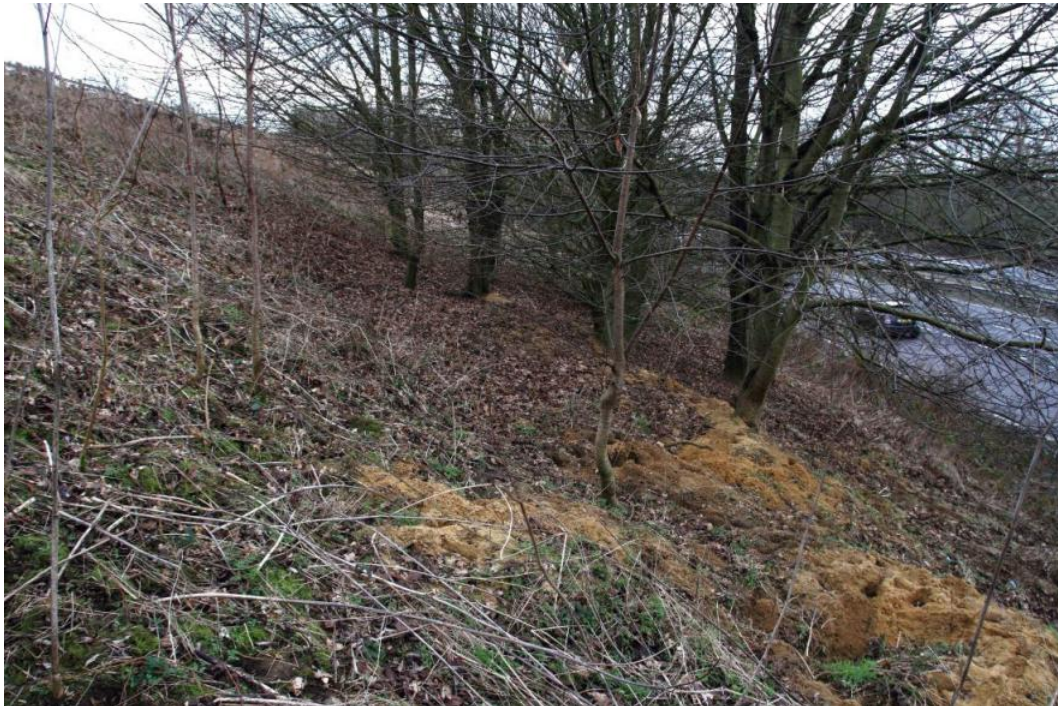
Figure 3: Area to the south of the trial at the A10 Hoddesdon showing signs of instability and badger activity (Site Photograph 7DW_4076)
