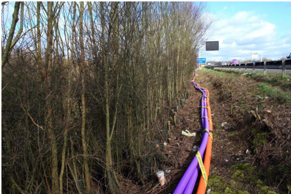
Figure 17: M23 Gatwick trial showing communications trench (to the right of the purple/orange conduits) and the remains of the willows that were removed during its installation. View to the north from the south end of the trial site (Site Photograph 7DW_4234)
